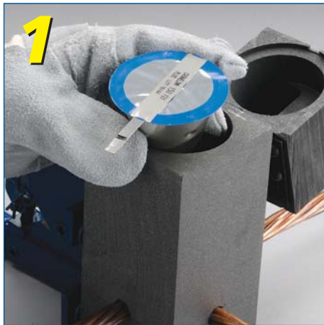
1 Insert CADWELD PLUS package into mold (may require use of a cover/baffle)
